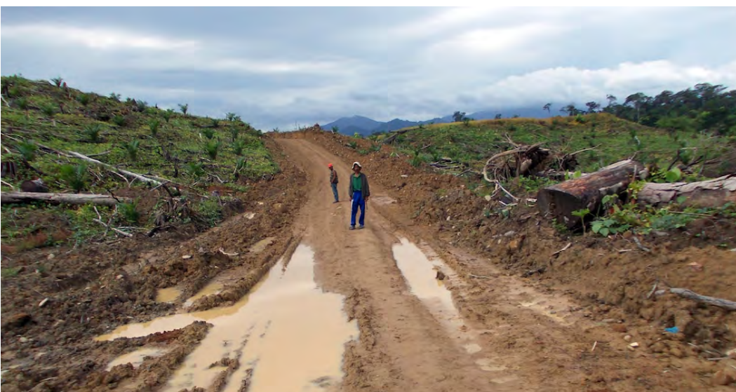
Illegal road construction by Agumil in Calasaguen (Municipality of Brooke's Point)
